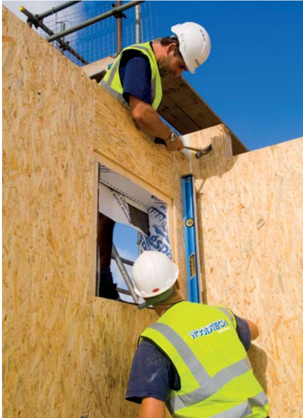
During 2012 the manufacturing of the TEK Building System structural insulated panels was moved to Selby.
